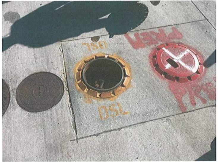
Photo 2: View of the diesel spill bucket before replacement
