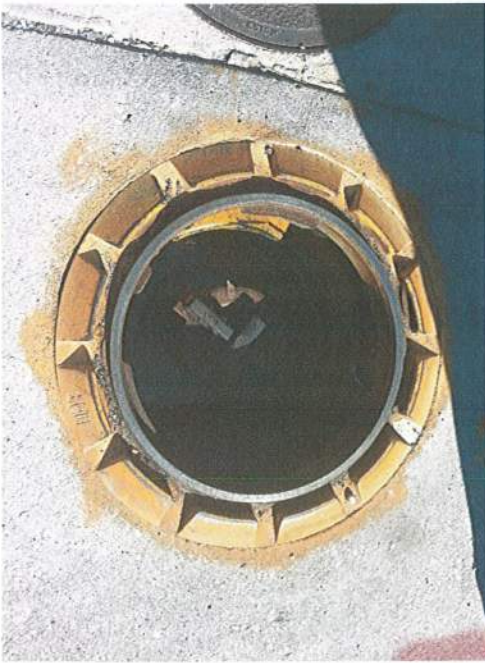
Photo 1: view of the diesel spill bucket before replacement
