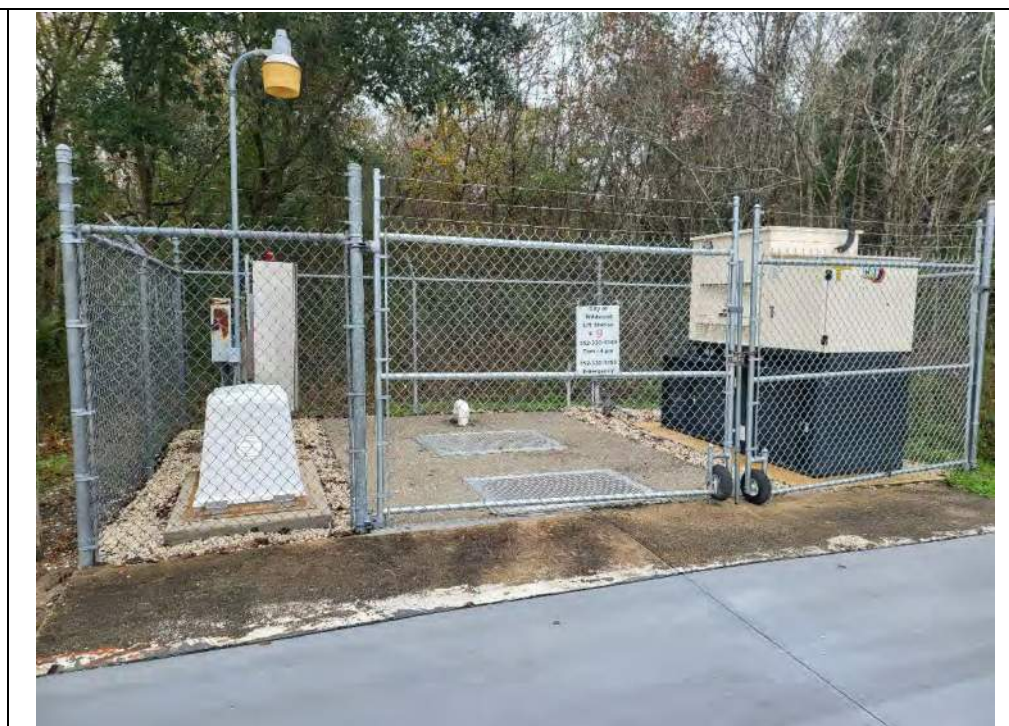
Looking east at the lift station and emergency generator belly tank.
